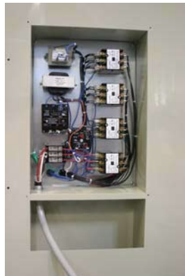
Electrical panel with contactors, transformers, compressor time delay, and phase protector.
